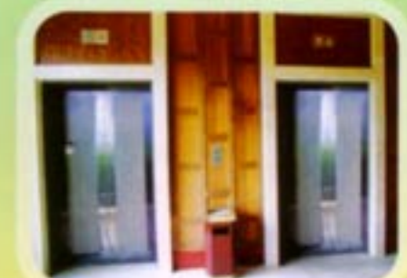
Passenger Service Lifts
